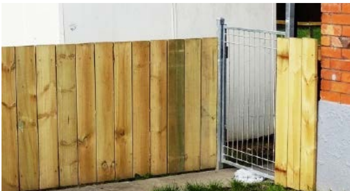
We are installing secure fences like the one above to separate play areas from driveways.
